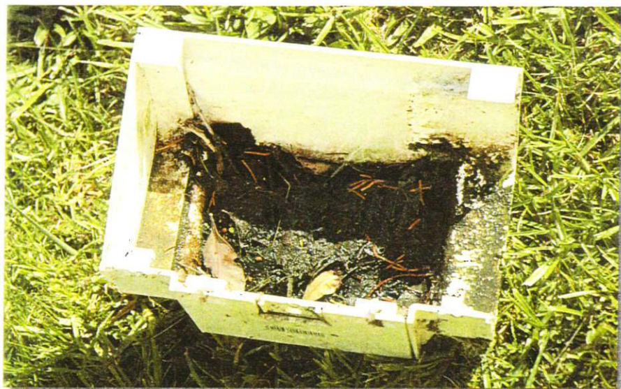
Gunge collects in unprotected gutter rainhead.
