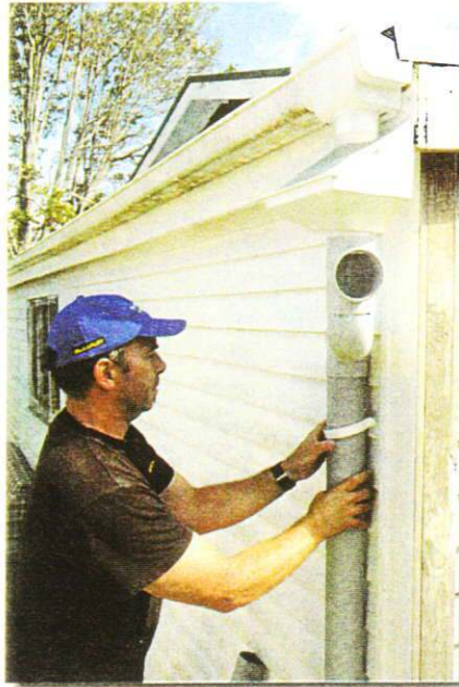
Fix elbows for downpipe first flush diverter,
